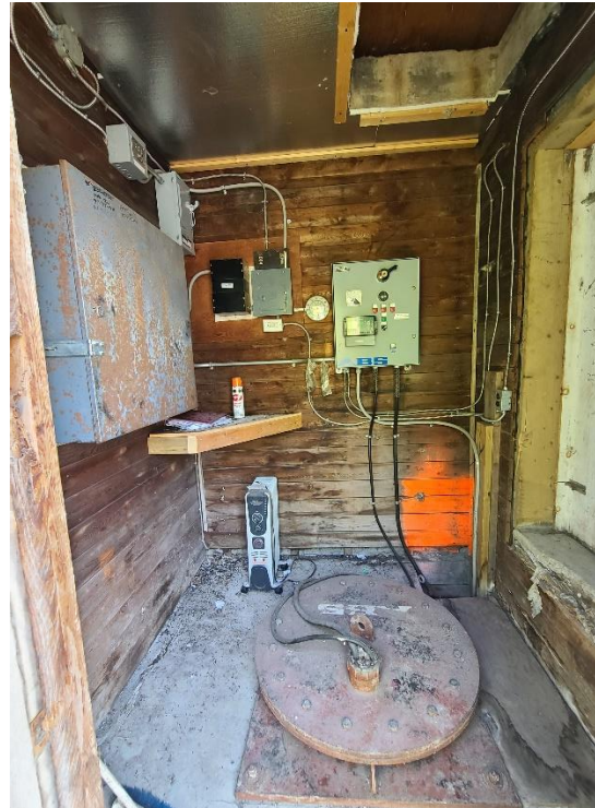
Figure 2 Interior Showing Pump and Controls
